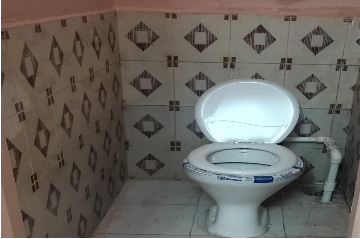
Toilet for Divyangjan
