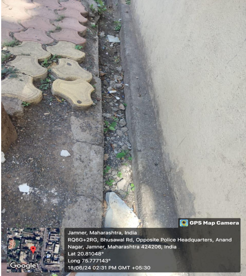
Outer Water Drainage
