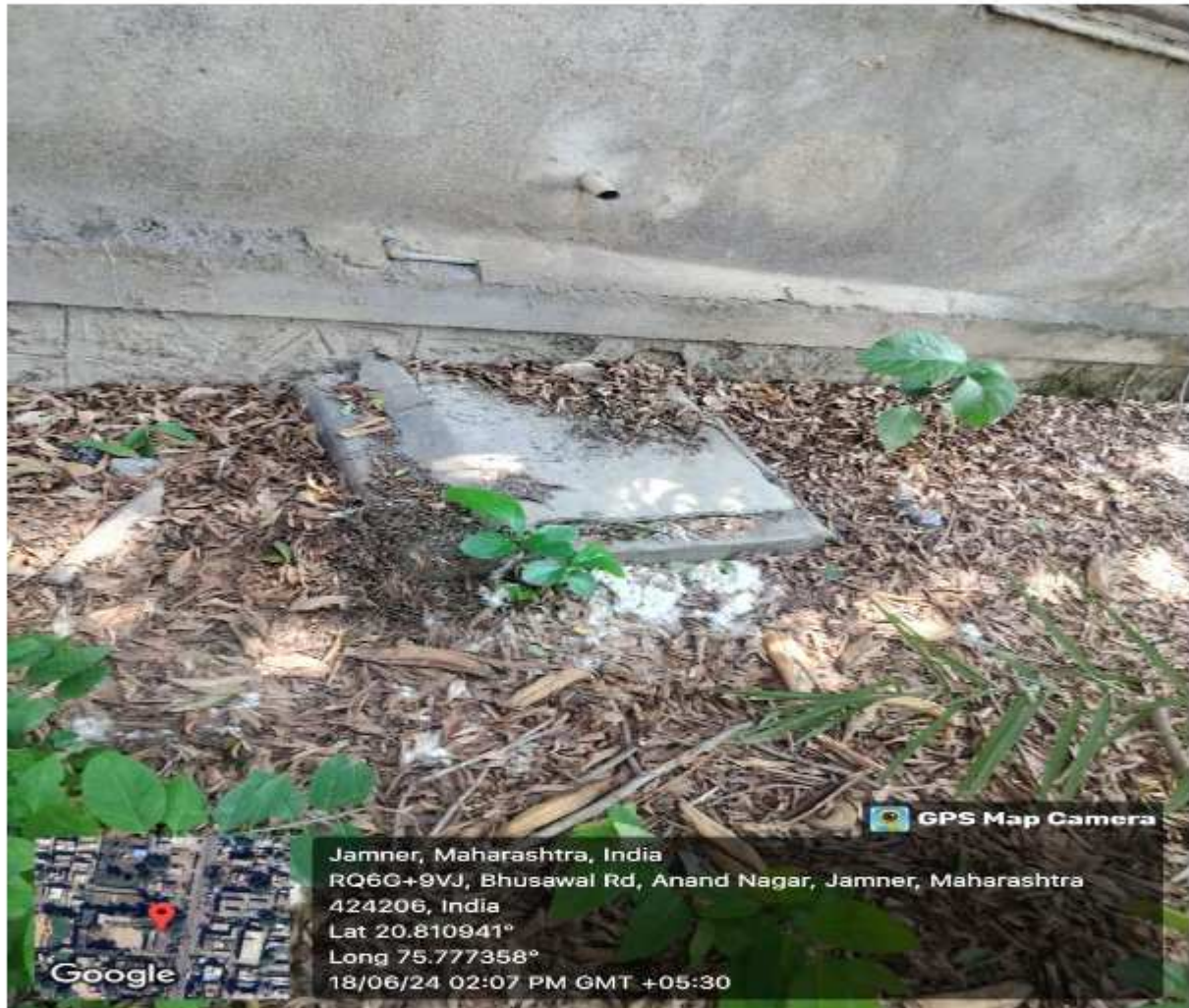
Toilet Water Waste Management Tank
